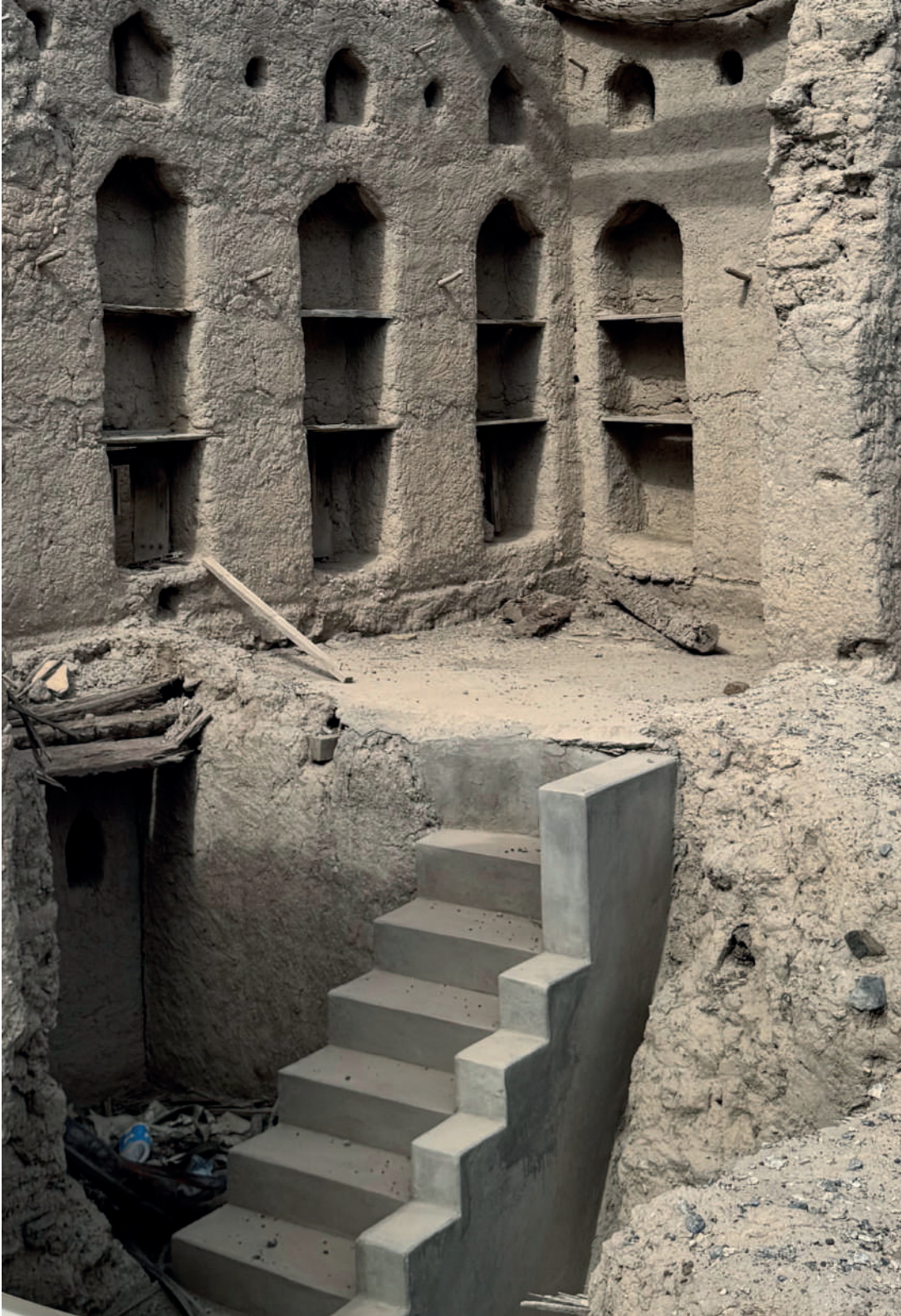
[5] Showing the combination of existing building ruins against new additions (staircase in concrete).
